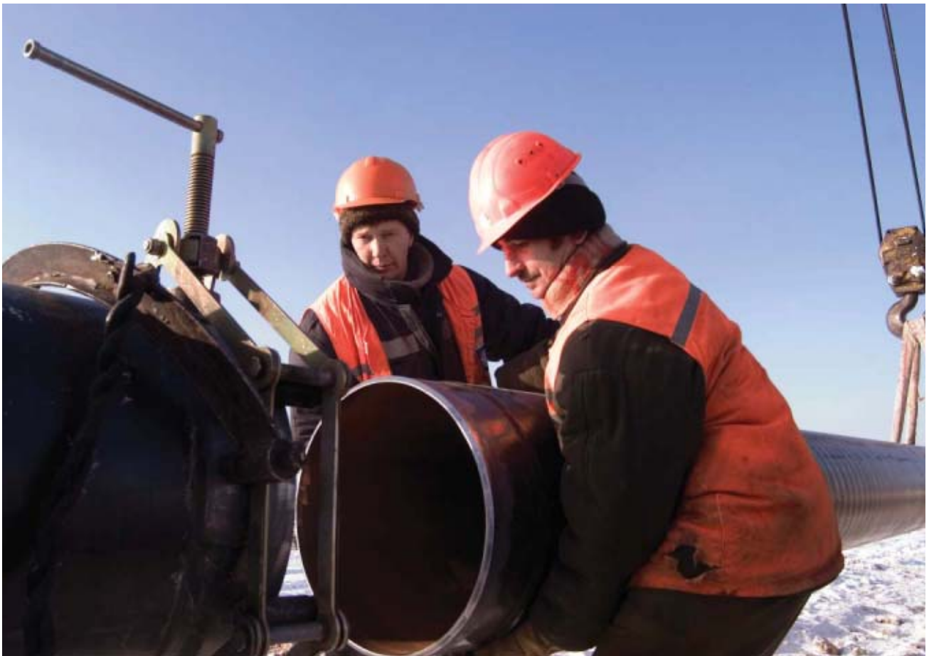
Pipeline integrity becomes an increasingly important issue with the dramatic expansion of facilities around the world. Here, workers connect line pipe in Salyng oil field near Salyng, Russia. Photo courtesy of Shell Photographic Services, Shell International Ltd.
